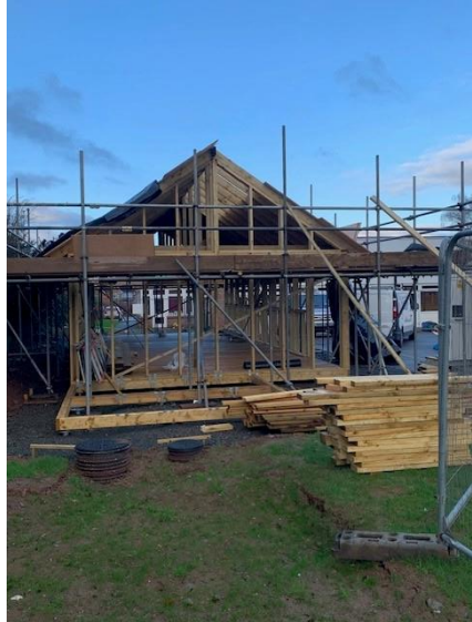
Clehonger CE Primary School – Demolition of mobile Classroom and installation of new outdoor classroom
